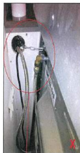
Hole in cabinet too large, Allowing the upright oven to tilt forward
