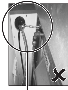
Hole in cabinet too large, allowing the upright oven to tilt forward
