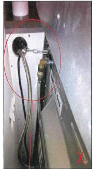
Hole in cabinet too large, Allowing the upright oven to tilt forward
